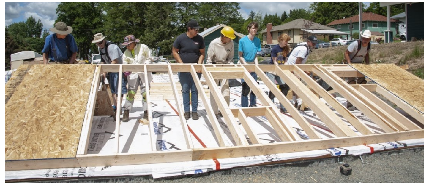
The Tara Lew Interiors Team with the Codger Crew raising the east wall of the Poulsen home.
