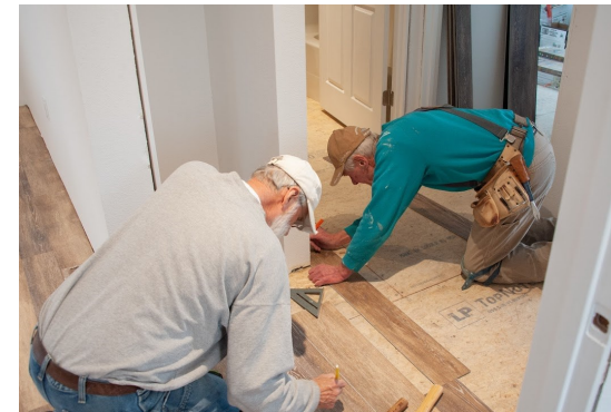
Codger Crew members Roger Willemsen and Dan Hardesty installing flooring. This flooring was specially selected to handle the impact over time from wheel chair use.
