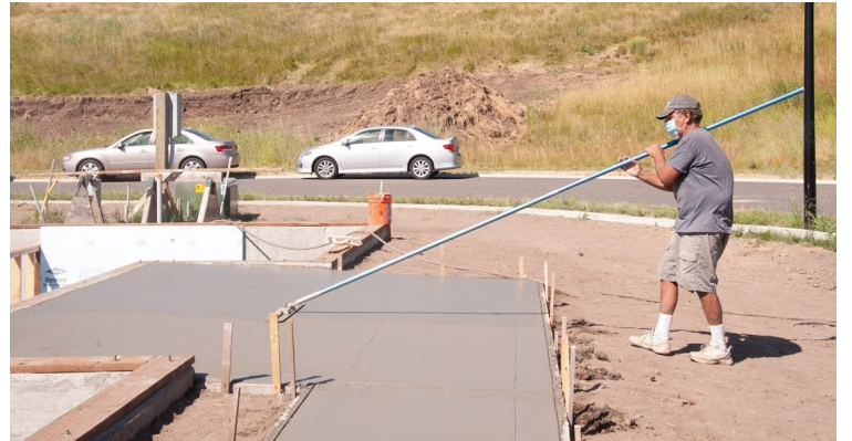
Construction Supervisor Dave Stradley puts the finishing touches on concrete poured at the Uniontown home.
