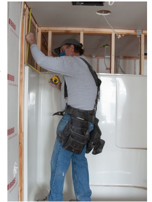
Construction Supervisor Dave Stradley measures for a piece of sheet rock in the master bath.
