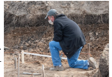
Construction Supervisor Dave Stradley checks the layout for the footings for the Hansen home.
