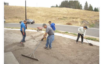
Dave Stradley prepares the Leaseburg yard for hydroseeding with help from future homeowner Kyle Hansen, and LDS service missionaries Elder Slaughter and Sister McKee.
