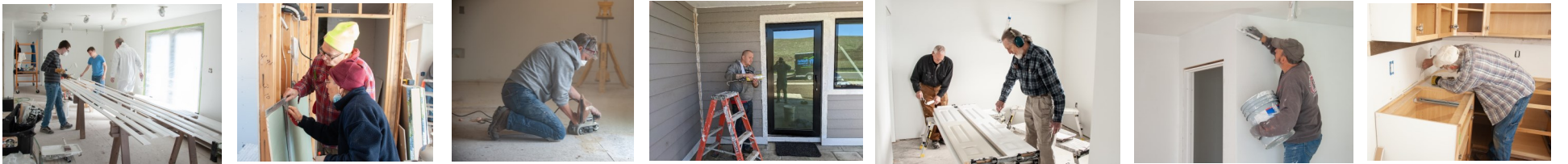
LDS Service Missionaries Elder Slaughter and Elder Carnahan paint baseboard with Jim Fredenburg. Codgers Carolyn Adam and Tom Gooch cut drywall to size. Codger Chris Montfort sands the subfloor to prepare for flooring. Future homeowner Kyle Hansen helps complete exterior caulking. Codgers Michael Haseltine and Jay Hunter paint closet doors. Courtney Smith paints edges. Codger Dan Hardesty repairing drywall after kitchen cabinet box installation.
