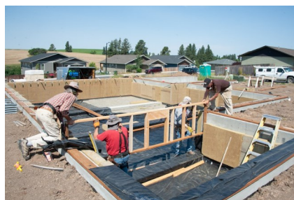
Top Row left to right: Slocum Excavation preparing for the foundation. Codger Crew members lay vapor barrier, install rockwool insulation to condition the crawlspace and place stem walls.
